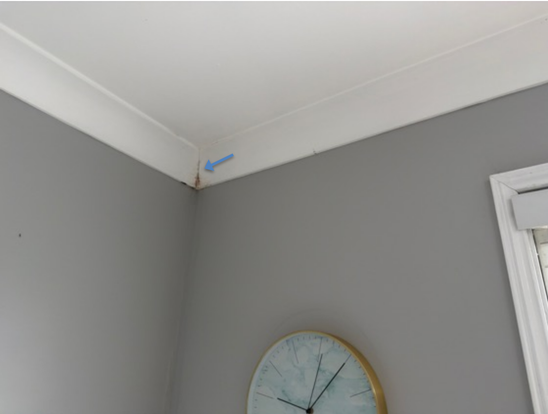
Cornices have past water staining.
