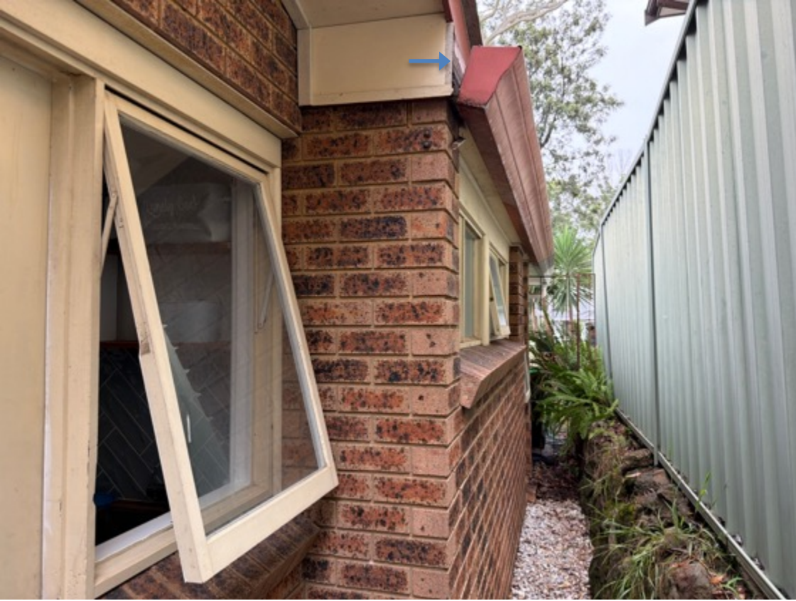
The left side elevation gutter requires remedial works.
