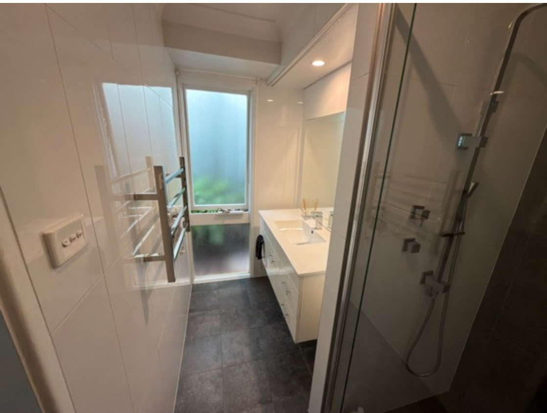
The ensuite bathroom area tested for leaks, fixings and stability was all clear at the time of inspection.
