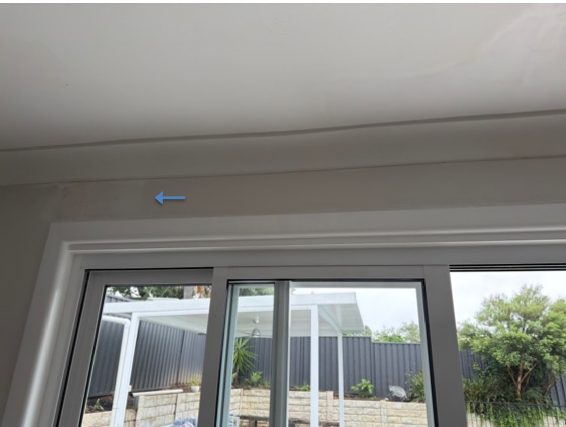
Internal painting works are incomplete, consistent with age.
