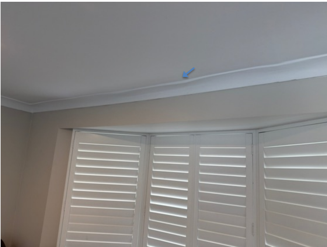
Plasterboard and cornices display imperfections – appear wavy (lower level television room example above.)
