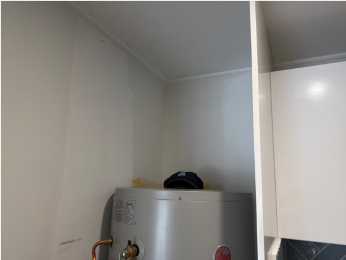
Painting works are incomplete in the laundry.
