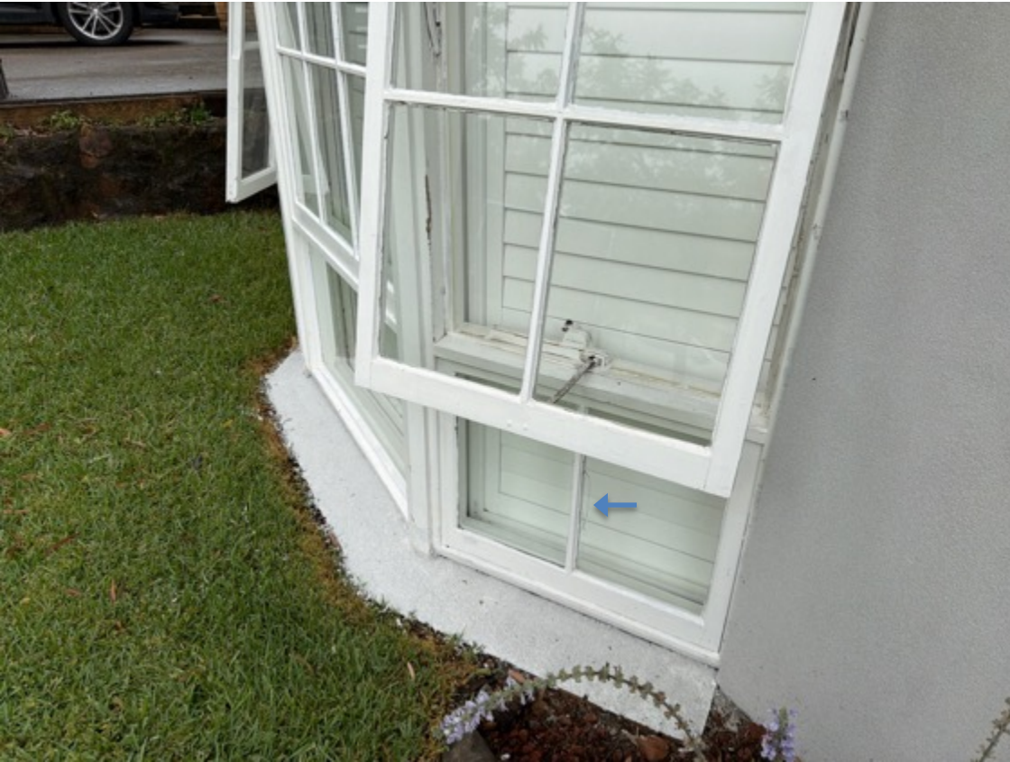
The front left window glass has a minor crack here.
