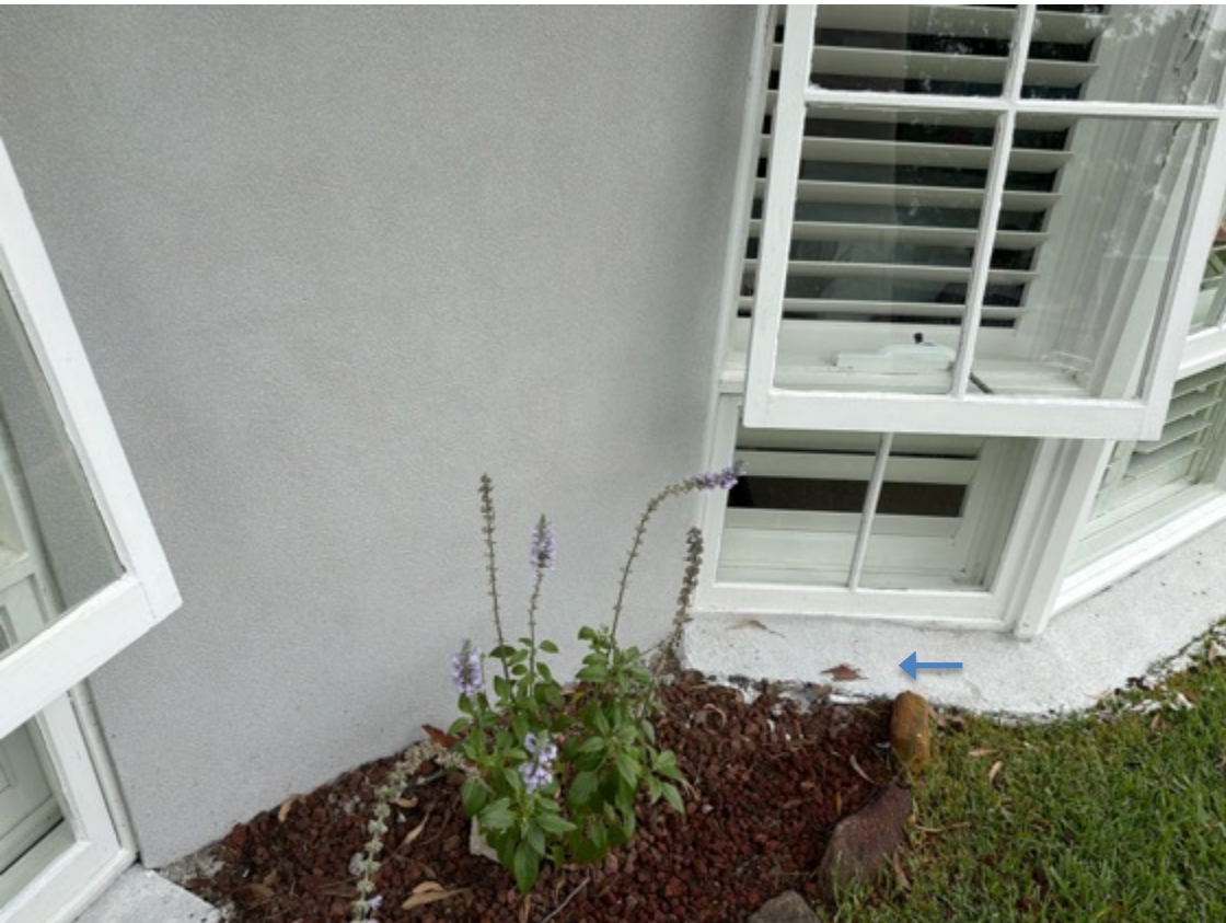
Isolated sections of external render is cracking and has minor damage, consistent with age.
