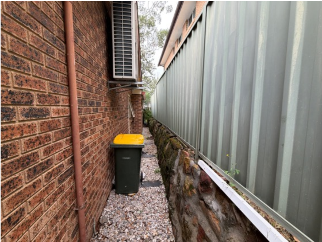
Site fences are in serviceable condition, isolated sections have minor damage and are leaning (consistent with age.)
