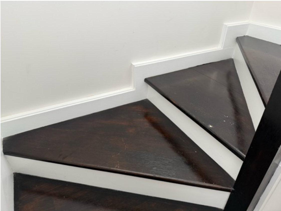
Sections of staircase steps feel uneven under foot.
