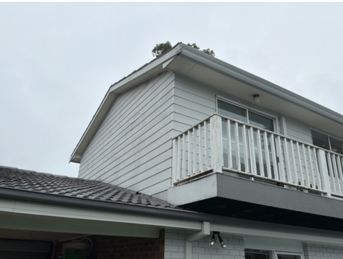
Exterior timber displays moderate to heavy signs of weathering – the rear balcony will require remedial works.
