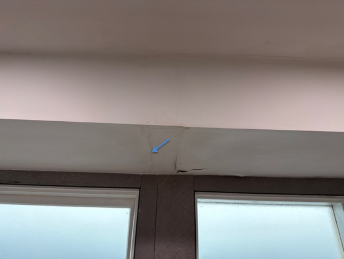
Plasterboard has past water damage visible here – will require remedial works.
