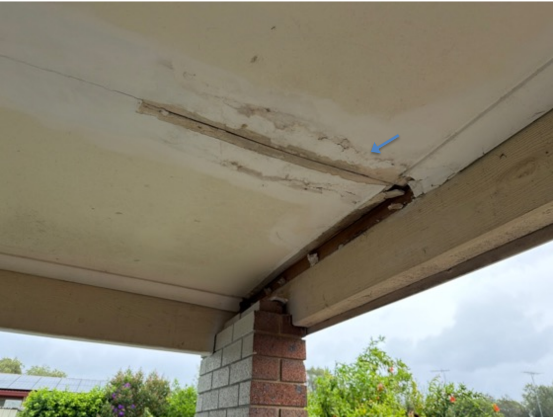
Plasterboard has water damage visible and works are incomplete (cornices, painting etc.)
