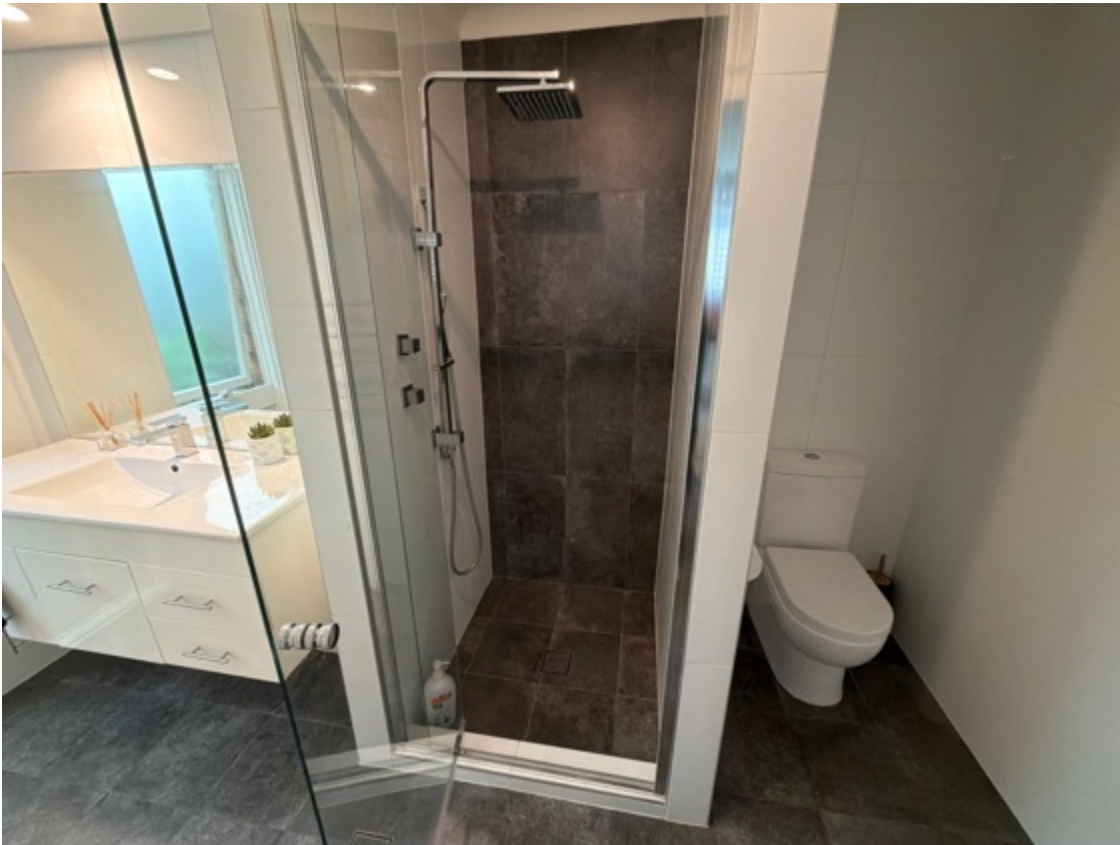
Hot and cold water services tested, functioned as intended at the time of inspection.
